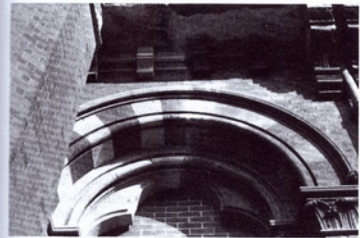
Figure 8.36 Successful cleaning with proprietary chemical products is quite feasible, but must be based on proper investigation and diagnosis of the cleaning problem, and not on a 'hit-or-miss' basis influenced by a particular range of products available. In general, more applications of material diluted down from the supplier's recommendations will achieve a better standard of cleaning. Very dilute hydrofluoric acid formulation was used to clean the flush banded brick and stone of St Pancras Station, London, with excellent results
