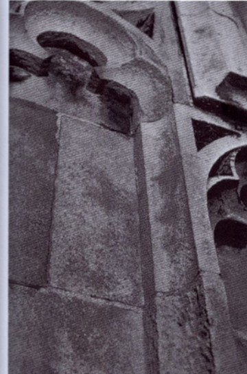
Figure 8.34 Failure to remove certain cleaning agents successfully can result in disfigurement or damage, or both. This illustration shows staining and efflorescence resulting from residues of sodium hydroxide left in limestone detail. Salt crystallisation damage is likely as wetting and drying cycles promote the distribution growth of sodium salts
