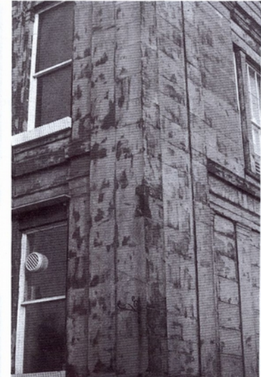
Figure 8.35 Failure to remove hydrofluoric acid will result in the formation of colloidal silica bound to the surface of the stone. This illustration shows carefully applied hydrofluoric acid formulation permanently bound to sandstone after being left for over twelve hours instead of 5–15 minutes. This disfigurement could only be removed by spinning, blasting or otherwise redressing the masonry to remove the outer 2 mm
