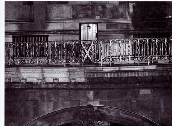
Figure 14.13 South transept, west wall, St Paul's Cathedral, London, England (Courtesy: Feilden & Mawson)
