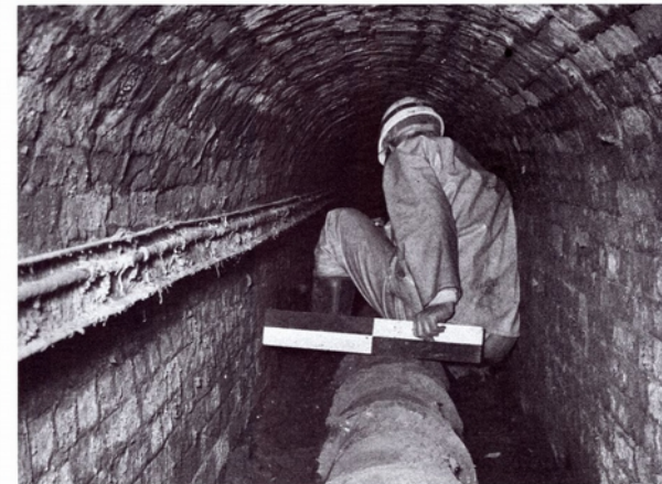
Figure 14.11 Original rainwater disposal system, St Paul's Cathedral, London, England (Courtesy: Feilden & Mawson)
